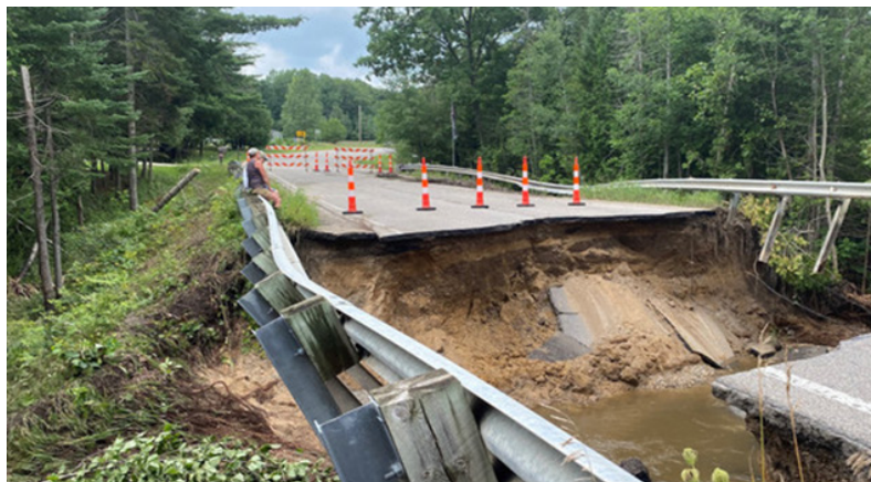
Image 1: Alden Highway Washout, Antrim County, August 2021
