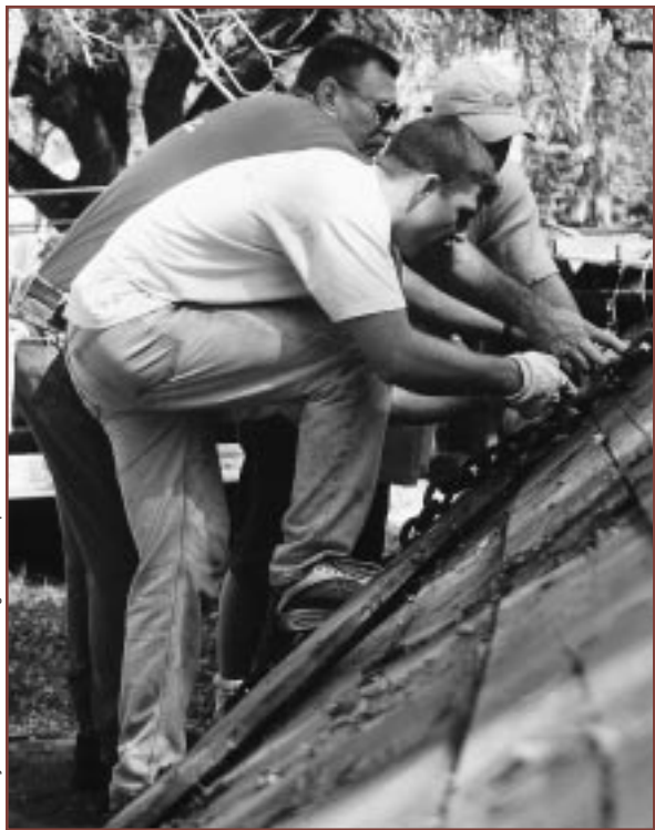
ROUGH ROOF. Doug Davis (center), rehab specialist at the Jacksonville Housing Partnership, and two U.S. Navy volunteers join hands to demolish an old shed for Jacksonville’s Paint the Town During Rehab Week.
