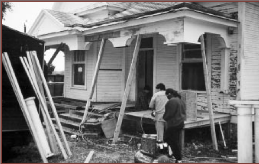
(Above) YEOMAN'S SERVICE. Rehab workers in Waco prepare to attack the overwhelming job of recreating what will become a beautifully columned porch.
