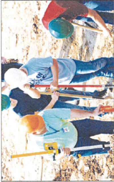
ALEXANDER SINI/CADILLAC NEWS CTC Applied Construction Technology student Bobby Pierson, wearing the white helmet, and students set the foundation for a home that will take two years to complete.
